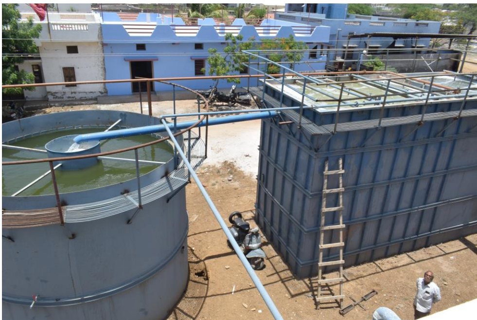
Fig.2: Secondary Clarifier and MBBR cum Aeration Tank
