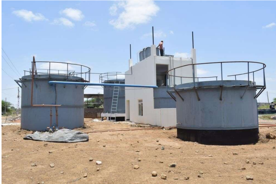
Fig.3: Secondary Clarifier & Settler-2
