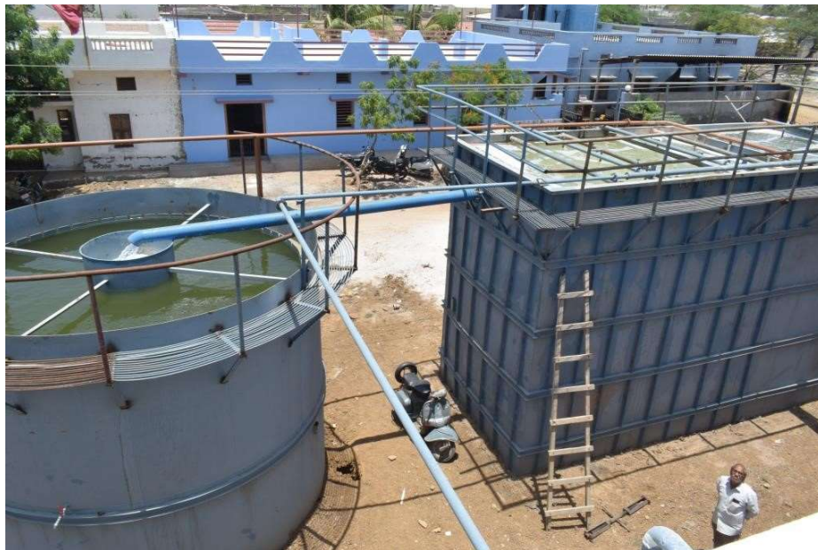
Fig.2: Secondary Clarifier and MBBR cum Aeration Tank
